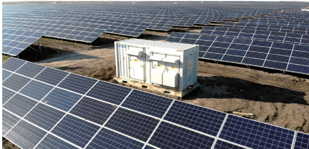
07 Utility Project in the Ukraine 200MW PV Plant
