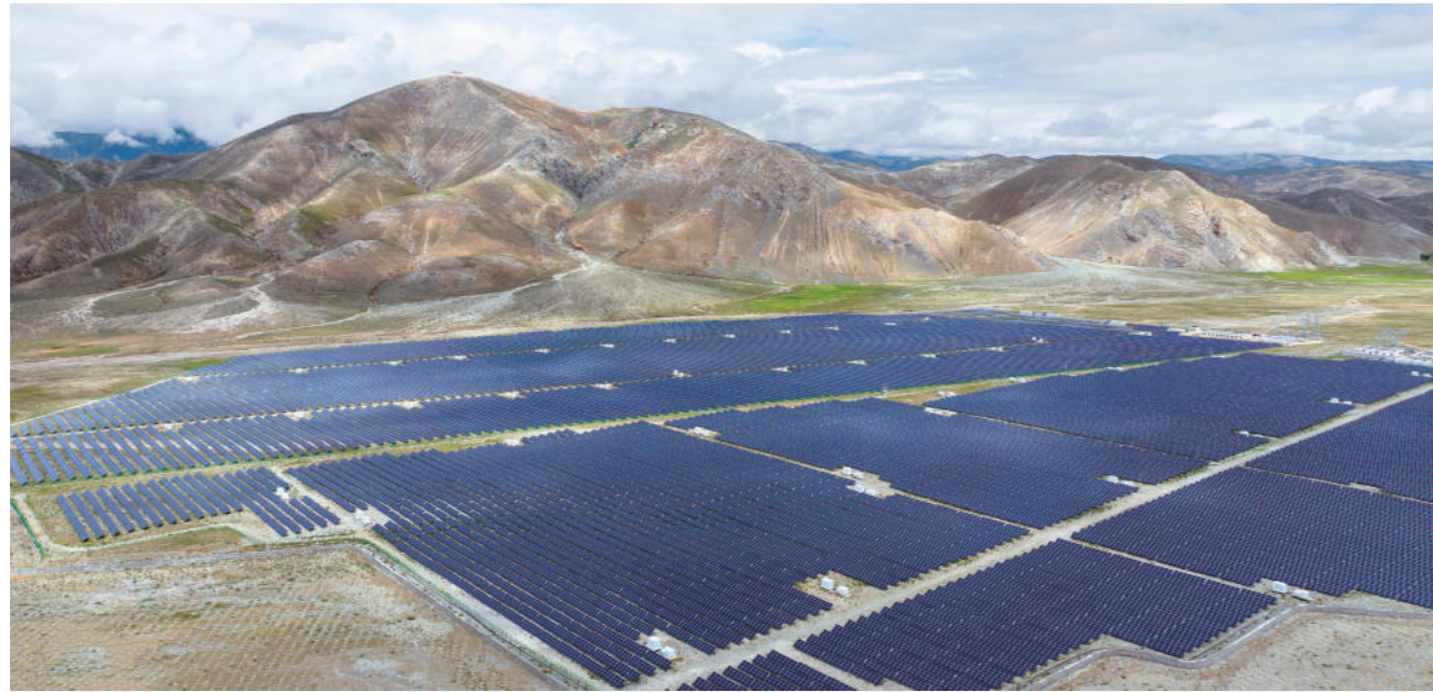
05 Utility Project in the Tibet 4747m Altitude PV Plant
